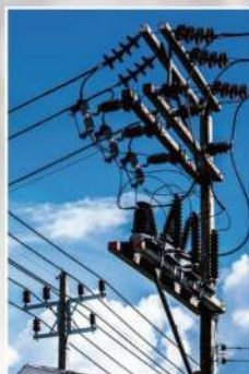
Power supply equipment
