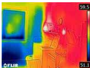
Uninsulated outside wall
