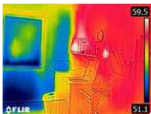
Uninsulated outside wall
